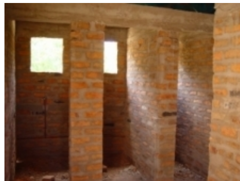
Shower Stalls in the Sanitation Block
